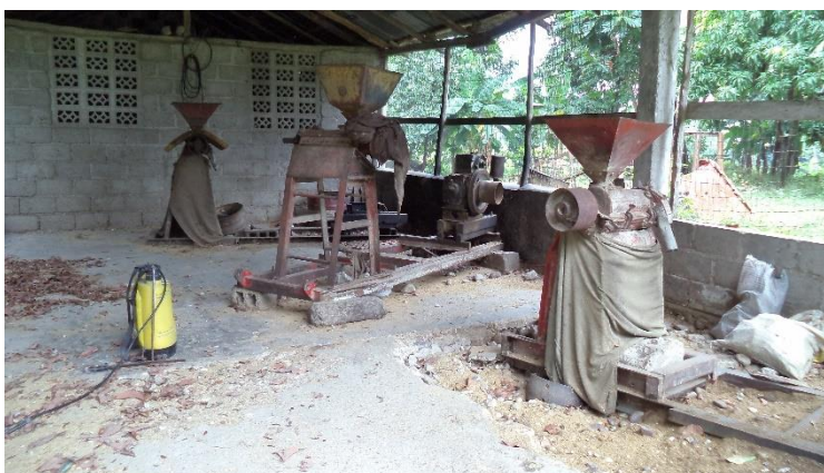
Axel's broken mills
