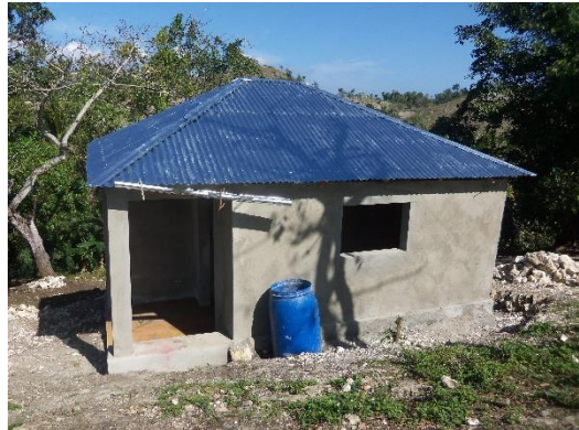
Figure 5: TTFB Breadfruit Factory under construction in Jeremie (not the same structure showed to the consultant on February 1 st 2018)
