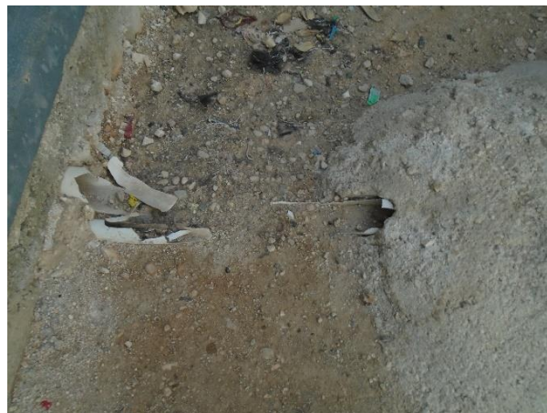
Figure F71: Broken septic pipe and septic tank.
