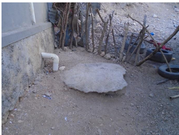
Figure F70: Pipe and septic tank.
