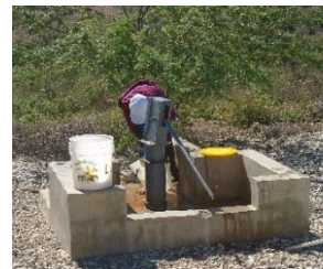
Figure F92: One of three wells.
