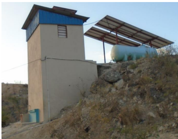
Figure F68: The Desalinizer, pump, and storage tank that according to residents has worked for three weeks of the past 5 years.
