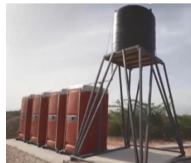
Figure F95: some of the showers and toilets
