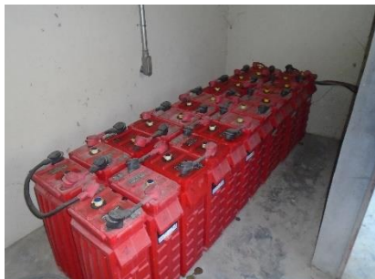
Figure F44: Battery bank that has not worked in over 1 year, at Lake Peligre Hatchery.
