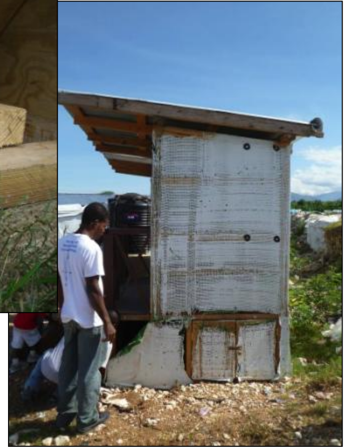
PHOTO BAD T9: Heat damage to plastic sheeting on side of SOIL UD toilet.
