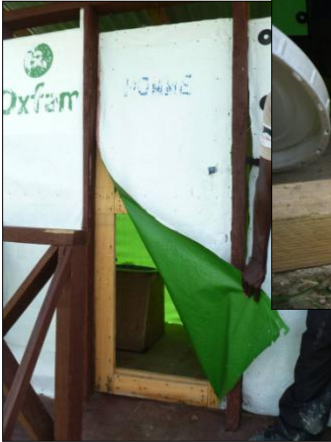
PHOTO BAD T7: Plastic sheeting deliberately detached by children, for access.
