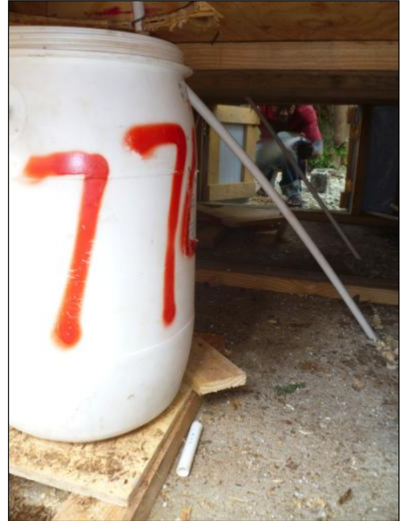
PHOTO T2: Drum in position beneath poophole
