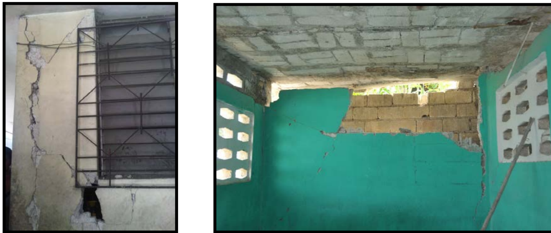
Fig. 03 – Shear cracking in wall pier (Left), Out of plane failure of CMU wall (Right)
