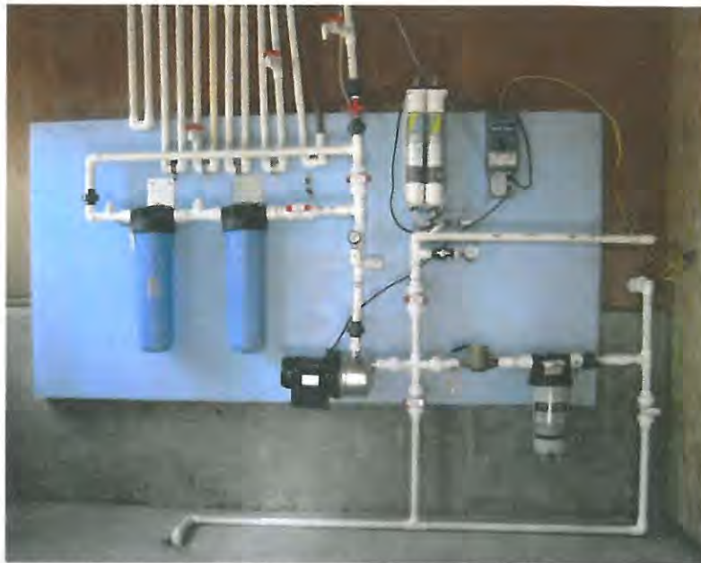
Clean Water U Bay 5 is an AC Ozone Disinfection System.
