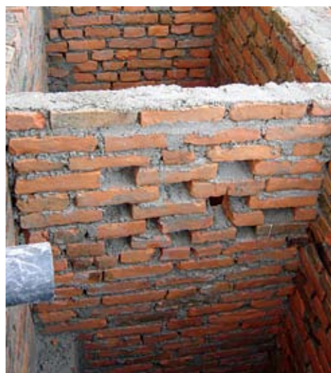
Poorly designed septic tank in a new house
