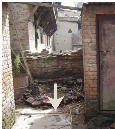
A single chambered tank with no provisions for FS emptying
