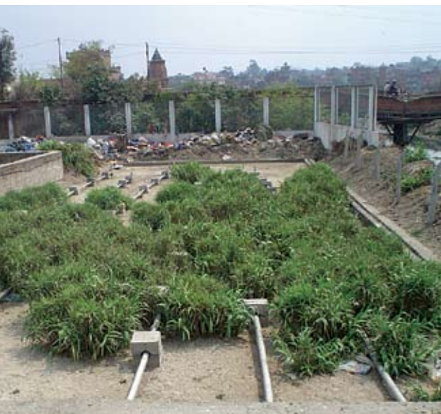
Teku septage treatment plant (non operational).
