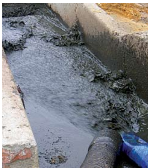
FS with high water content being disposed at Teku Septage Treatment Plant, Kathmandu
