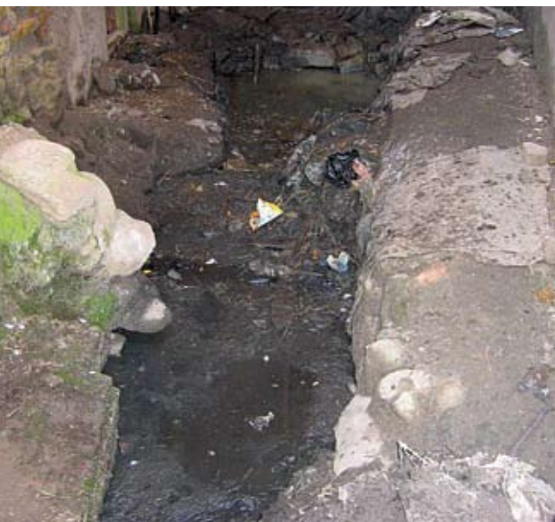
Wastewater disposal from household into open drains
