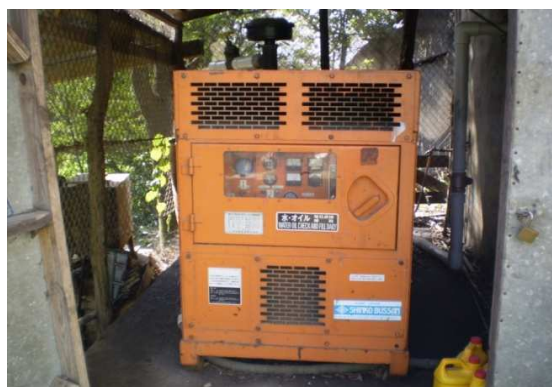
Biogas powered generator
